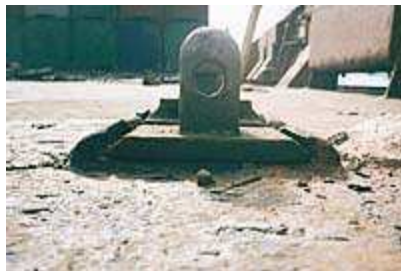
Photo 2 - Incompatible locating cone which is too small for deck fitting and can be removed vertically.
