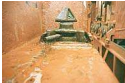
Photo 1 - Chamfered edge of deck fitting distorted sufficiently to allow twistlock to be removed vertically.
